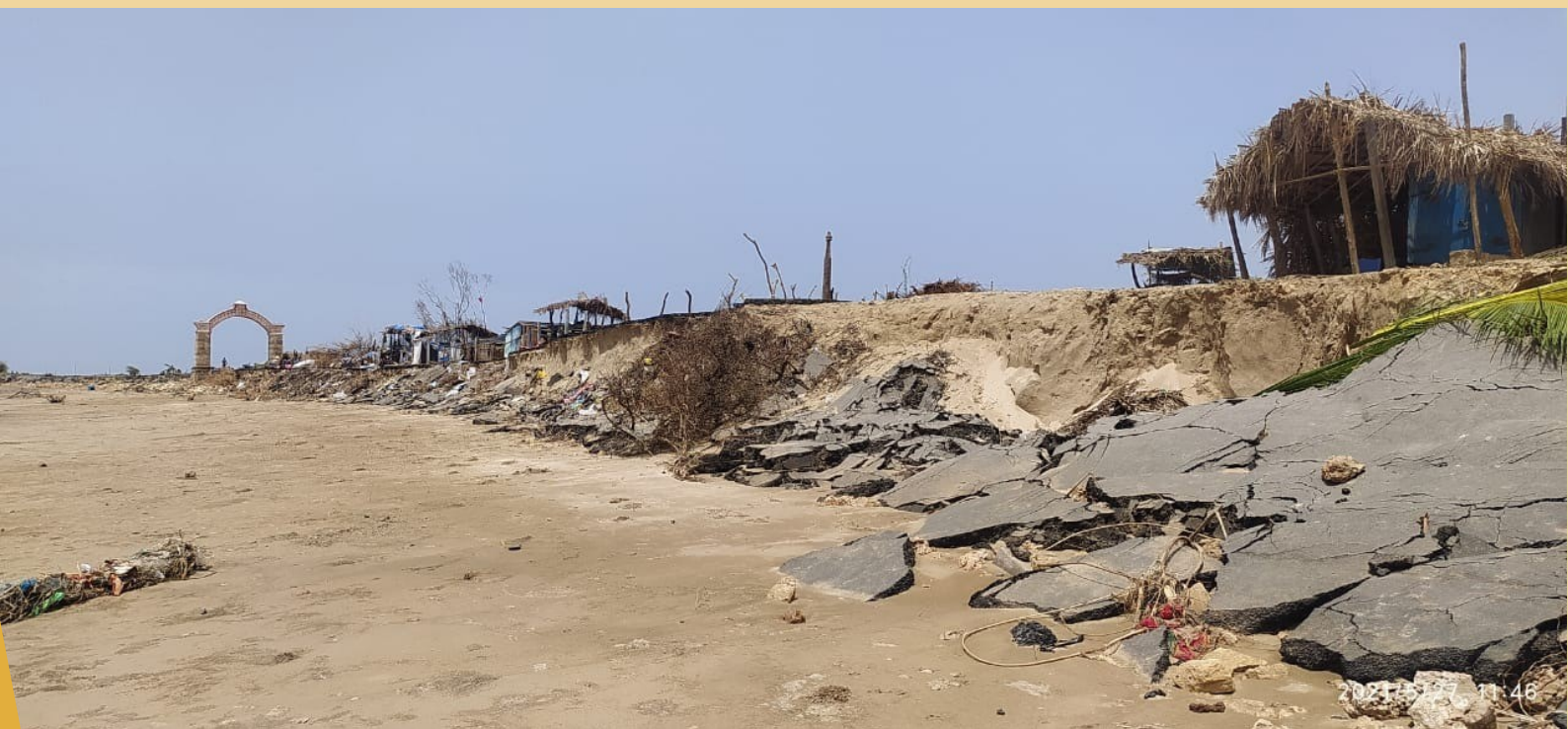
Newly constructed road along Simer beach (Port), washed away with 200 huts of fisher community.
